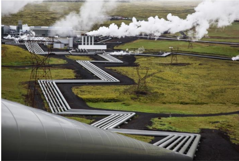
Giant ducts carry steam to the Hellisheidi geothermal power plant near Reykjavik, Iceland. (© AP Images)
