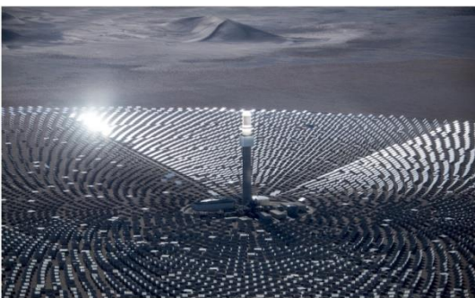
Mirrors track the sun, directing its energy to the receiver atop the Crescent Dunes tower. (Courtesy photo)
